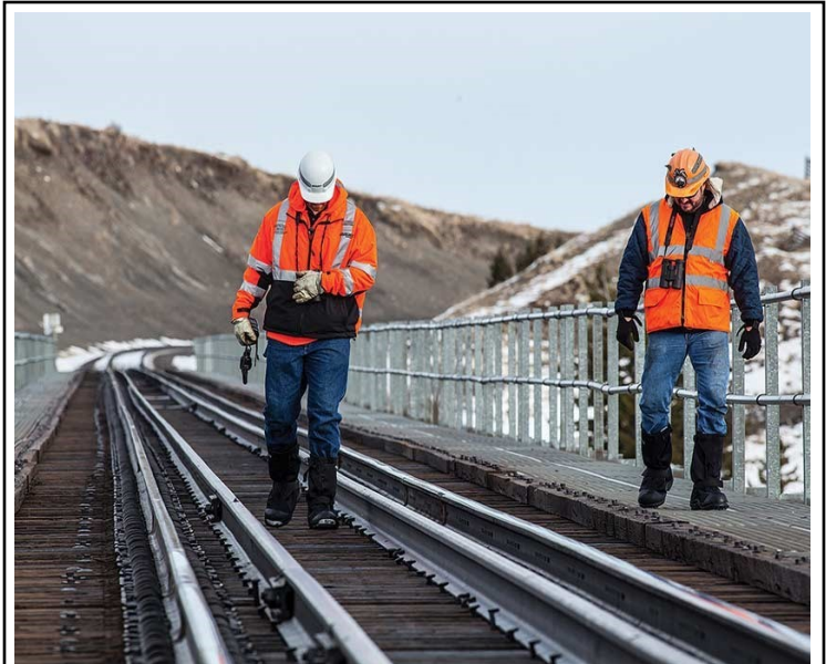
Maintenance-of-Way workers inspect a bridge in 2015. The crafts hardest hit by furloughs and layoffs in the last few years have been in maintenance and transportation. While thousands of car inspectors, track and signal maintainers, trainmen and engineers stand idle, the railroad industry appeals to the federal government for relief from adherence to certain safety rules due to manpower “shortages.” Rail unions are up in arms over these patently false and misleading claims that threaten national rail safety.
